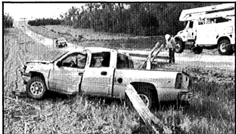
Crews work to replace a utility pole following an accident northwest of Wayne on May 14.
